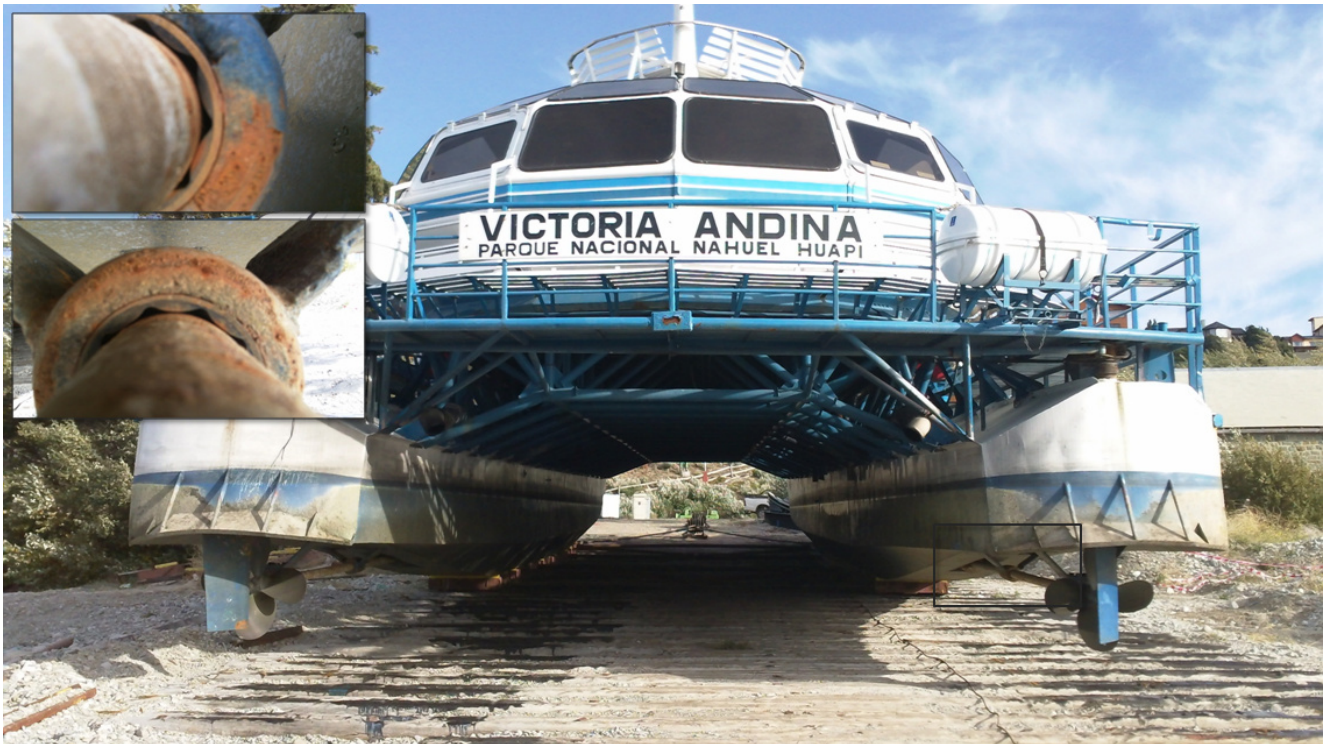
Figure 8: Detail image of corroded bearing-supports and worn rubber bearing-pads that carry the submerged tail shafts in the Catamarán Victoria Andina , identified in dry docks during 2012. Photos courtesy of Martín Pereira.
