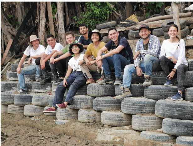
Figure 10. Retaining wall in used tires and construction section (2019) (source: Eduardo Peñaloza Kairuz and Brandon Ponce).
