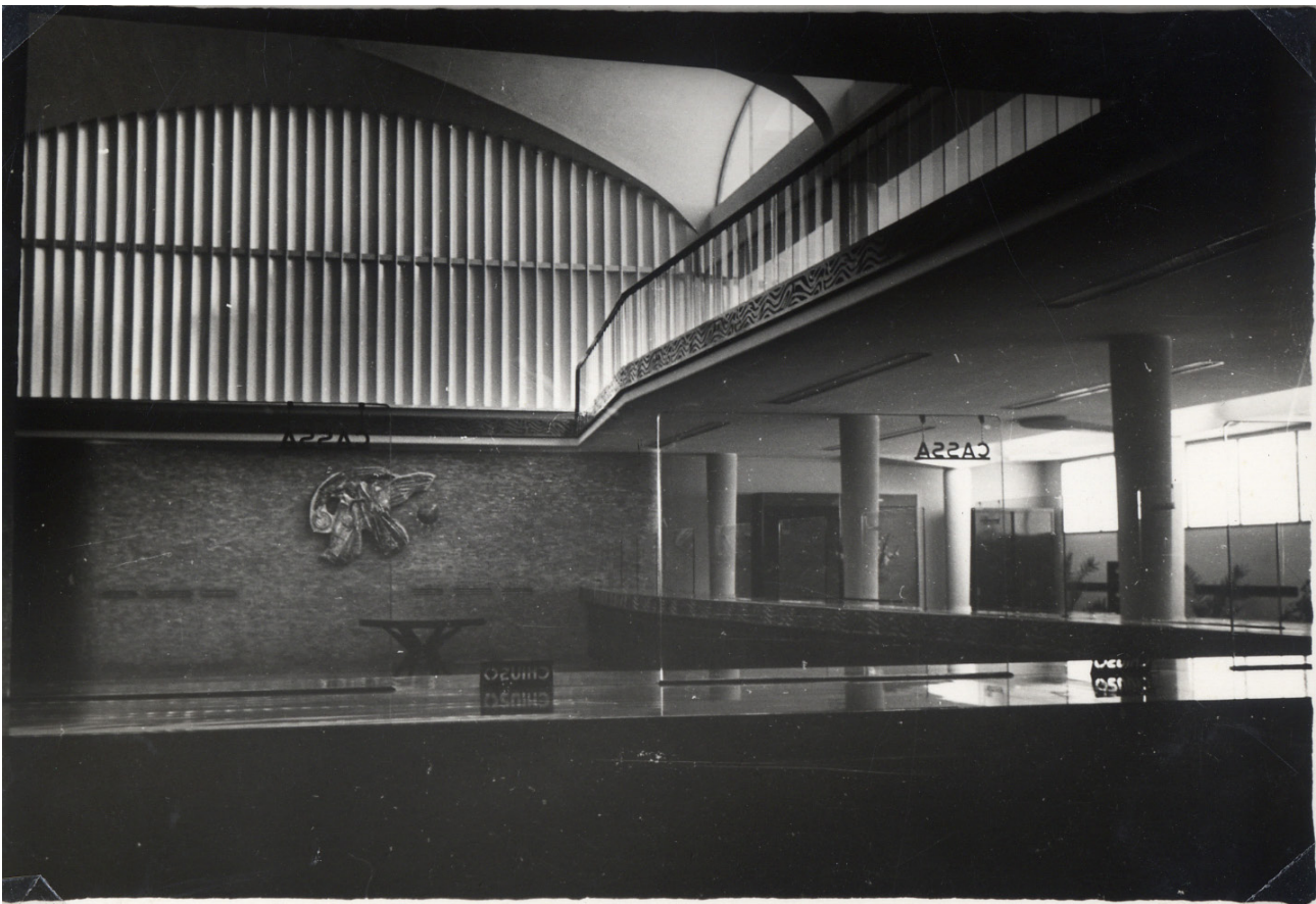
Figure 7. The Public Hall after work is completed. Note the lunette vault and the transparent wall with the sunshades where the stabilization tie-beams of the resistant system are inserted (source: Carispaq).
