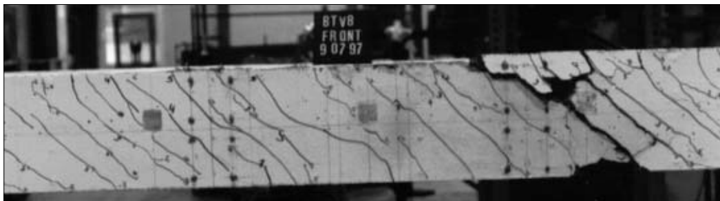
Figure 14d. Computed and observed crack development in the front web (BTV8)
