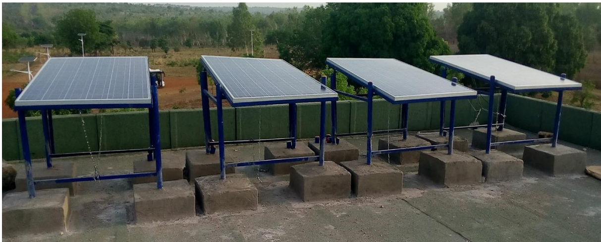
Figure 5: Photovoltaic field installed on the roof of the FaST
