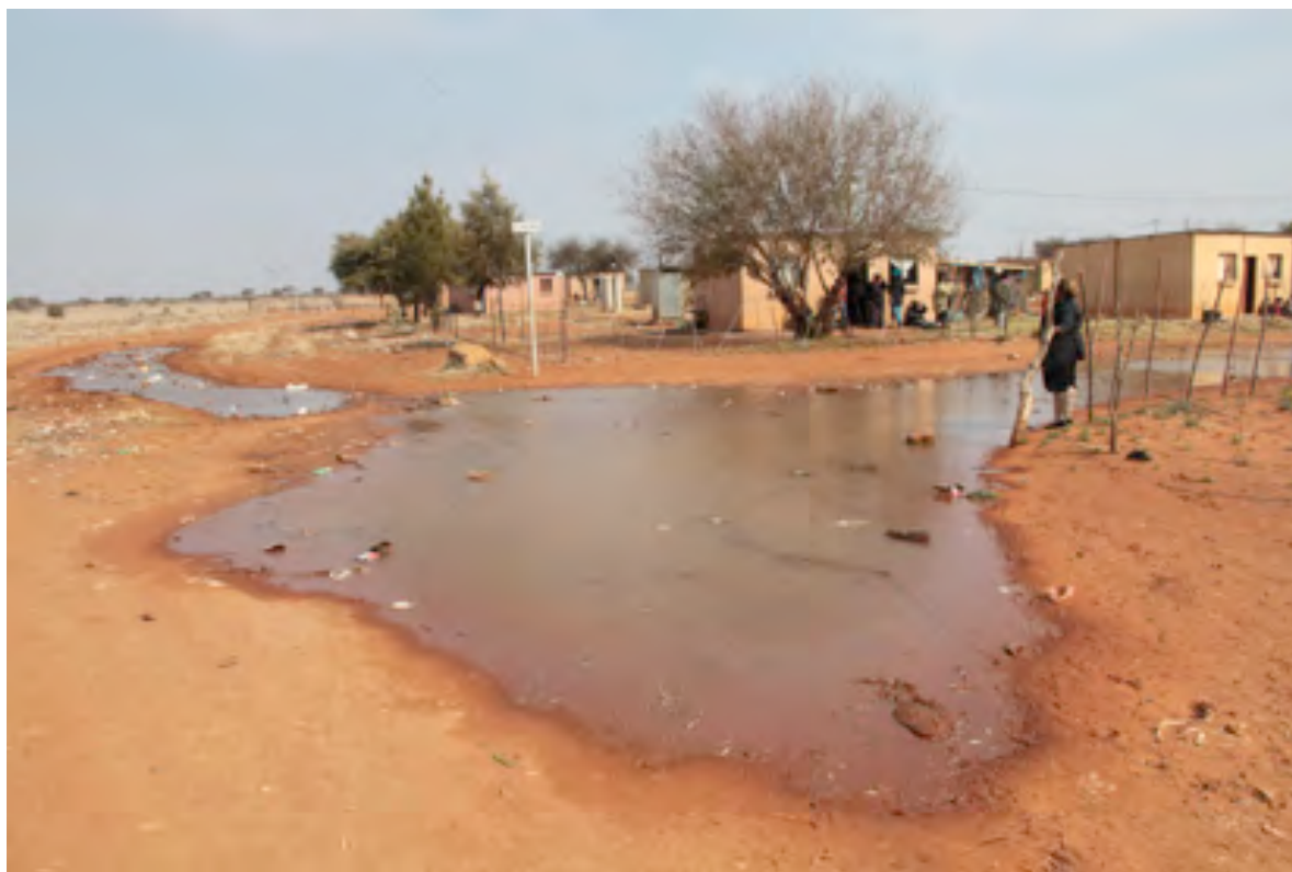
Figure 10 Motorists are unable to use the Chere Street T-junction road for fear of damaging their vehicles in the leaking water on site. (Photograph: JWN Tempelhoff)
