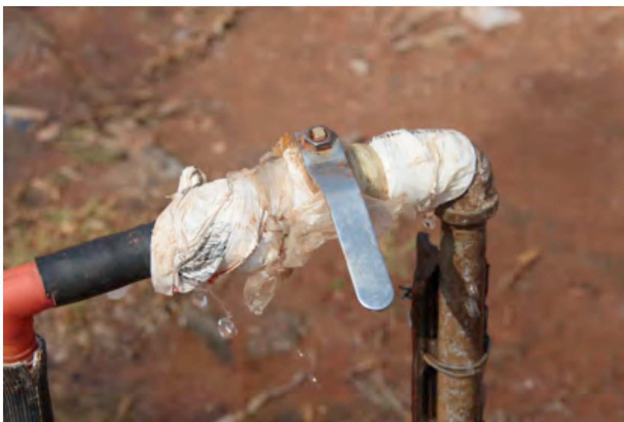
Figure 5 Some resident use plastic bags to stop tap leaks (Photograph: JWN Tempelhoff)
