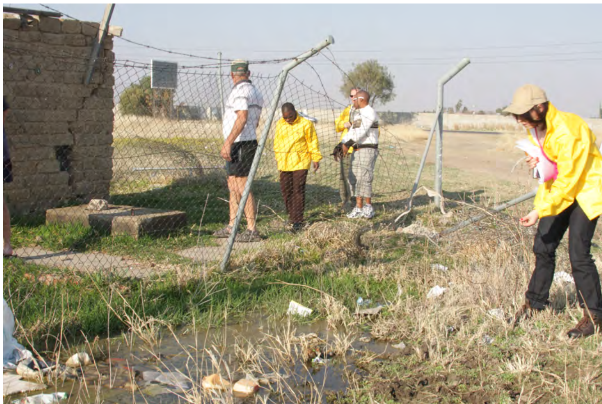
Illustration 1 One of the borehole pumping stations in the wetlands of the Harts River at Sannieshof in September 2009. The site had lots of rubble. The fence was damaged and the pumping house's walls badly cracked. (Photograph JWN Tempelhoff)
