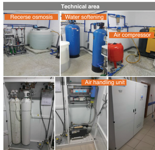
Figure 5: Typical technical installations in a CSSD
