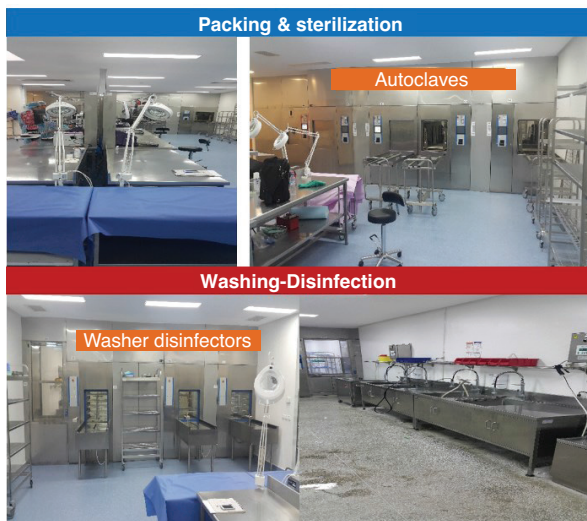
Figure 4: Main Equipment in a CSSD
