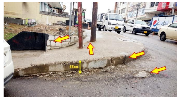
Figure 12. Poor sidewalk slope design and power poles configuration.
