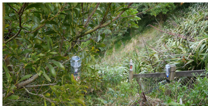
Figure 2: Moturoa Transmissions installation showing temperature sensor probe suspended left, ec-sensor attached to fencepost on the right and the base station further in the background
