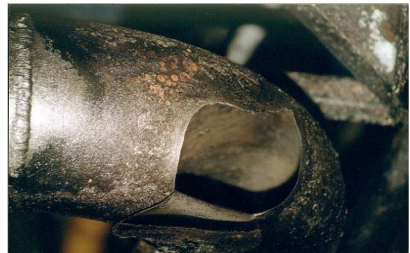
Fig. 3 A DN250mm tube broken by pressure a few weeks after the minor plant modernization.
