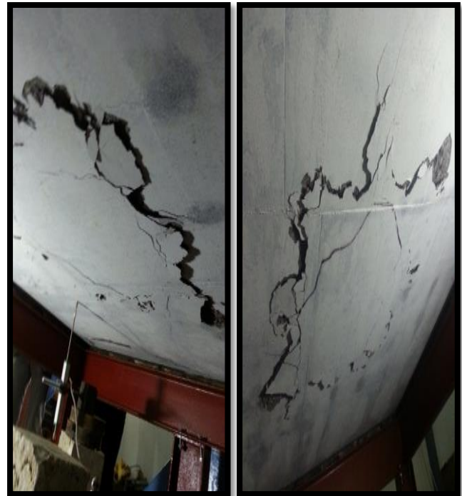
Figure 5. Crack pattern of selected tested slabs
