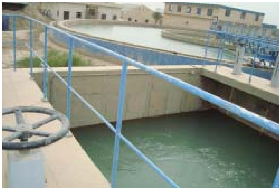
Figure 2. Coagulation and ClariFlocculator Tanks in DWTP
