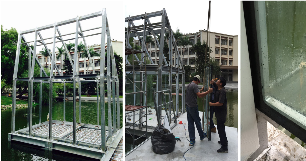
FIG. 9 Water House 2.0 during construction, showing the steel frame (left), positioning the panels (middle), and establishing the maintenance zone between floor and panel (right)
