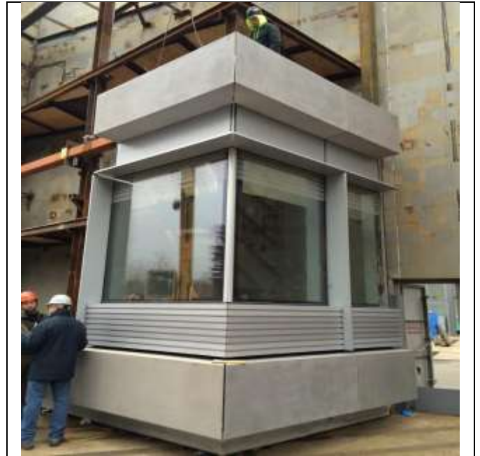
Full-size mock-up of the UHPC panel application for NYU's new Kimmel Pavilion
