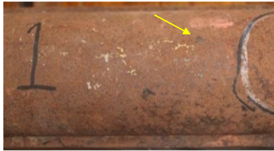
Figure 1.1 Pipe with damage (shown by arrow) caused by impact of foreign object
