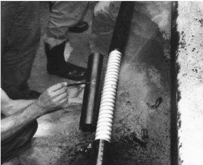
Fig. 4. Oil leakage found in the maintenance of the 138 kV transmission line Adelaide – Carlos Prates in 1997.
