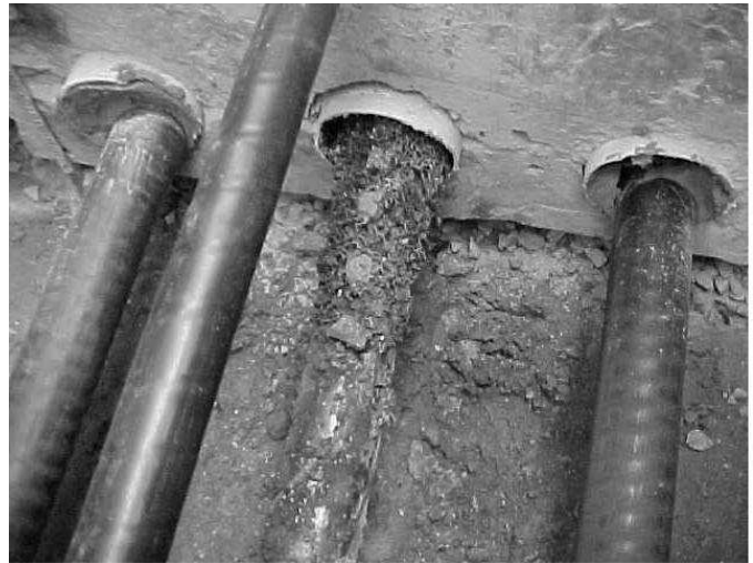
Fig. 5. Typical colony of termites found around the cables.
