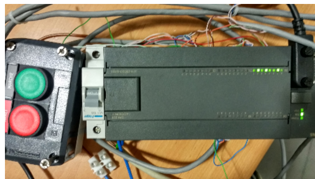
Fig. 6. The PLC and HMI
