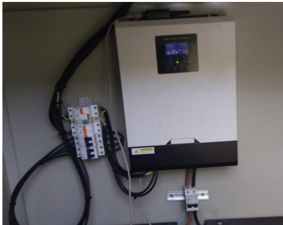
Figure 4. Solar electricity generating Inverter
