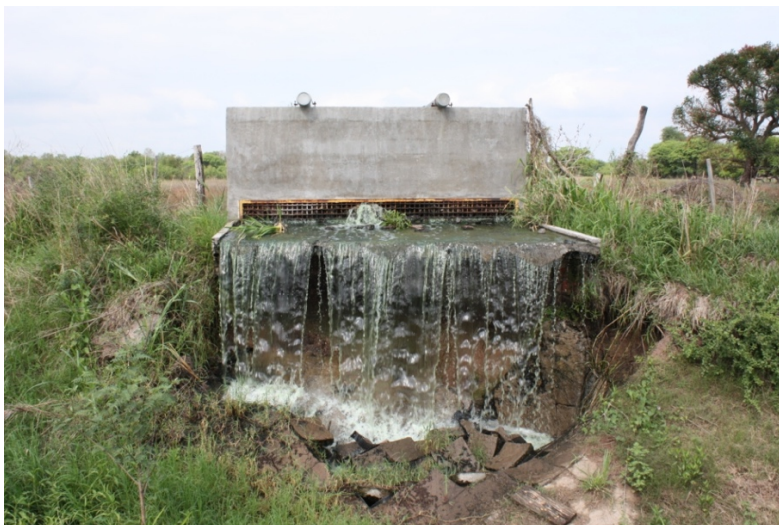
Figure 9. Ecological filter built to repair the environmental damage in Colonia Aborigen Chaco caused by sewage diversion from the neighboring population of Quitilipi. Photo by Author, 2010.
