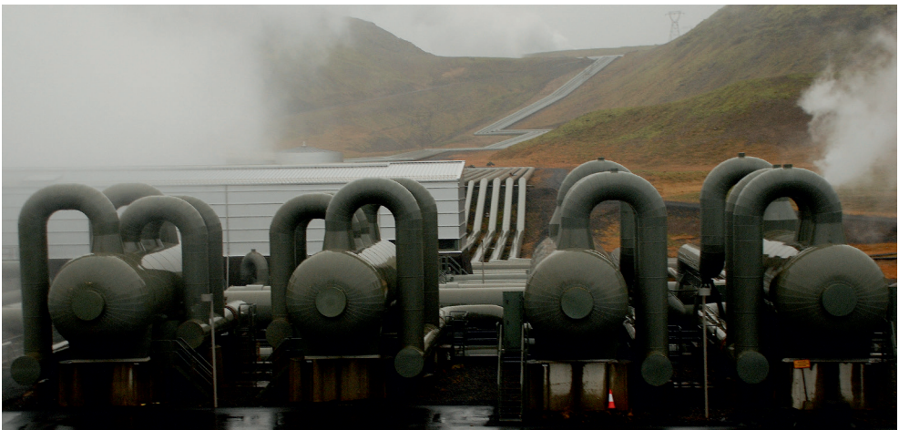
Photo 2. Hellisheiði Geothermal Power Station, Iceland (Photo by CENTER1, Cs.)
