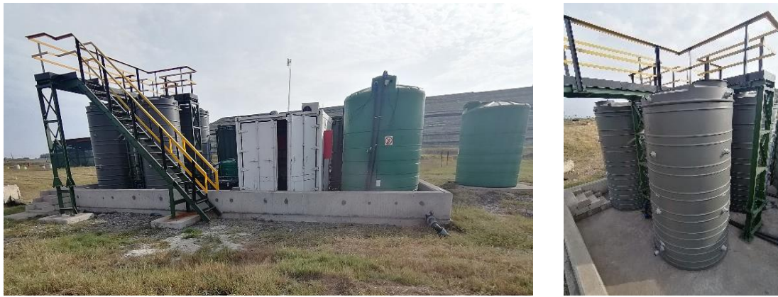
Figure 2. Semi-active pump and treatment plant implemented at site B, located in the North West province of South Africa
