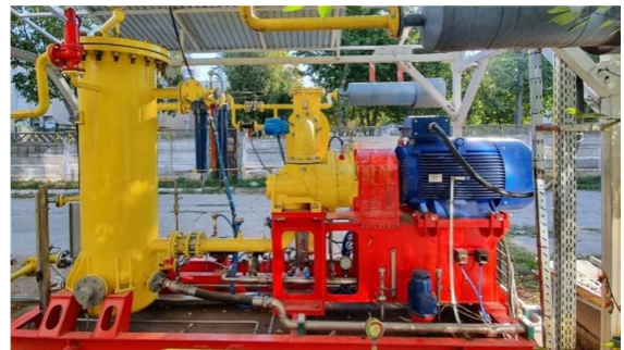
Fig. 1. Screw compressor installation.
