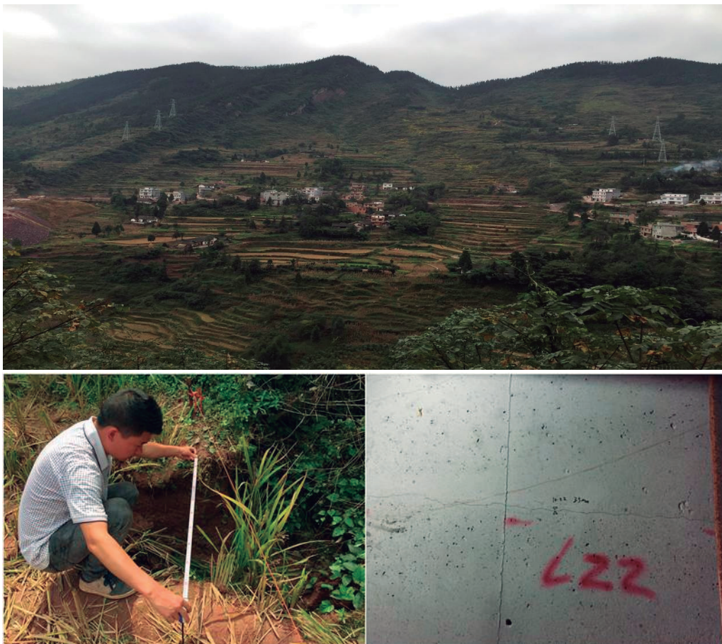
Figure 1. Deformation and cracks of tunnel landslide in Jimei
