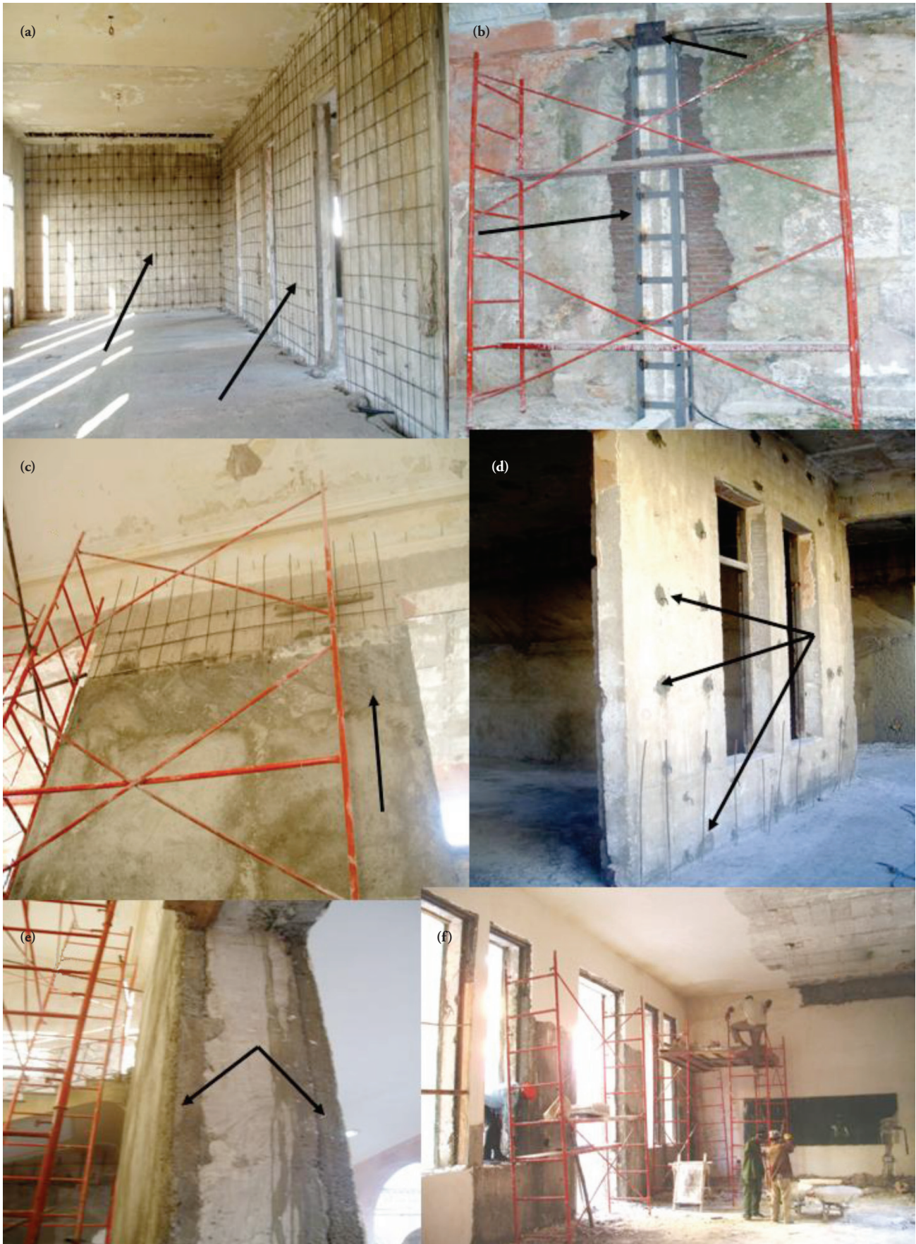
Figure 4. Structural reinforcement to increase seismic resistance in the Mendive project. Pictures courtesy of Francisco Calderín Mestre, project member.
