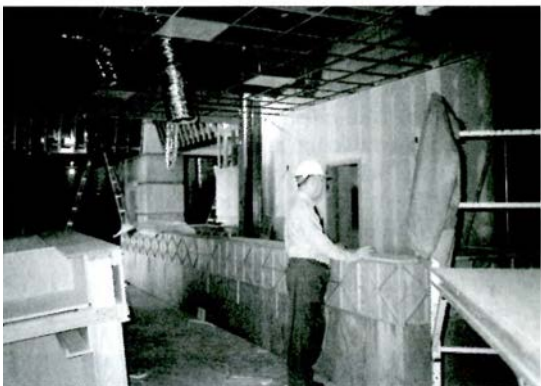
Take lots of photos to document progress throughout the project. 1) Feb. 1990—Reference Desk area, Eric and Sarah Rodgers Library for Science and Engineering, University of Alabama, Tuscaloosa.
