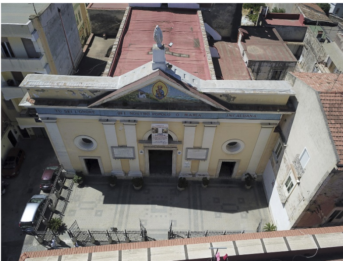
Fig. 1. Basilica Minore di Maria SS. Incaldana, drone view before restoration work (Ph: Antonio Smirne).
