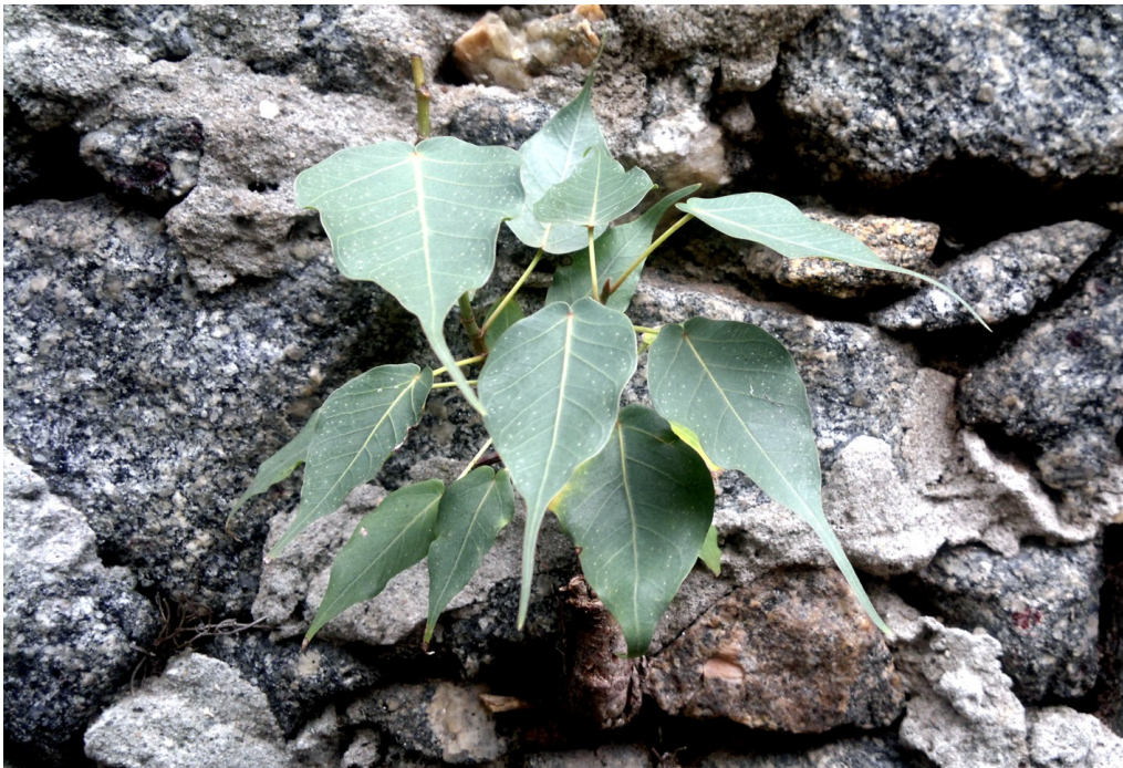
Figure 1. Plantlets of Ficus religiosa L. sprouting through a wall in Rio de Janeiro.
