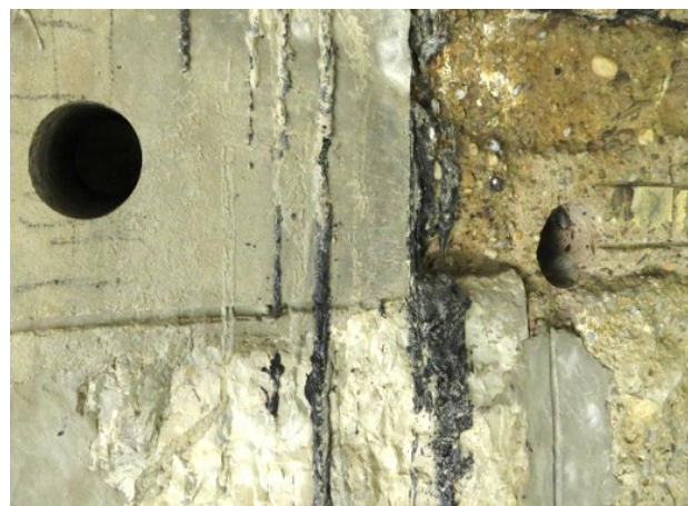
FIGURE 3. Places where drilled core samples were taken from the bridge abutment - on the left: the site with the protective render coat and on the right: the place where the render spalled over time (Bridge in Sládkovičovo).
