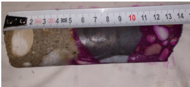
FIGURE 7. The carbonation depth of concrete at the places where this render was missing - sample selected from measurements performed in 2019 (Bridge in Rimavská Sobota).
