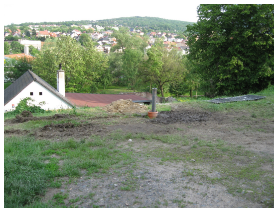
FIGURE 2. Temporary water pressure resistant steel casing of a borehole during realisation (located in an orange KG-System PVC sewage pipe backfilled in the manually dug trench).
