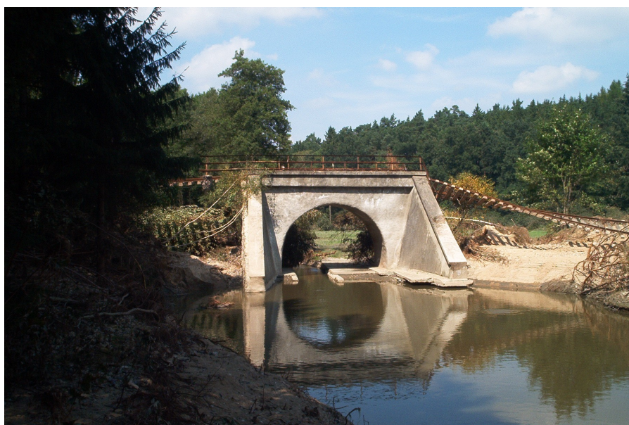
FIGURE 3. The erosion of Blatná – Nepomuk railway embankment. The water table shown on photo is typical for an ordinary flow rate.
