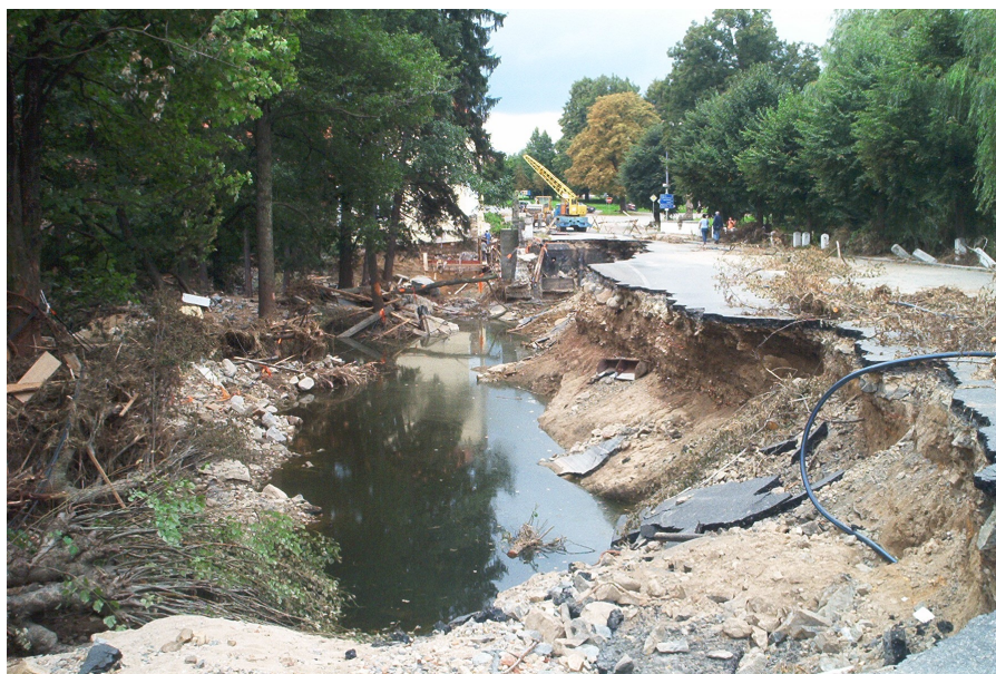
FIGURE 2. Example of disturbance of the downstream slope and crest of a dam which is used as an important communication line – E 49.
