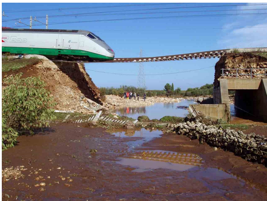
FIGURE 5. Failure of the railway track Bari – Taranto, 2005.
