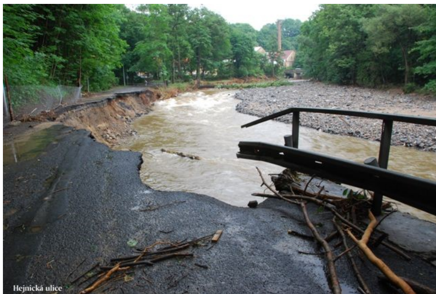
FIGURE 4. An example of lateral erosion of a transport embankment in the Frýdlant region, 2010.
