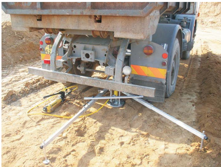
Fig. 3: Static modulus of deformation being measured on a layer of sand in the Klíčany sand pit
