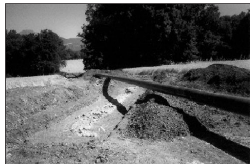
Fig. 4. Buried segment of the Roman aqueduct layout exposed by a gas company excavation.
