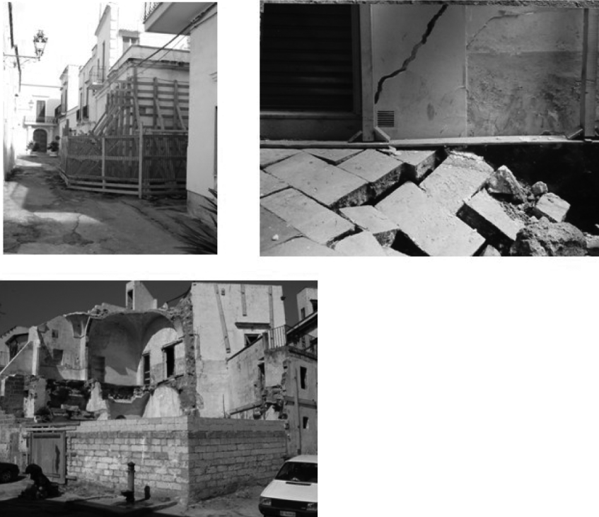
Fig. 1. Photos of soil subsidence in urban areas.
